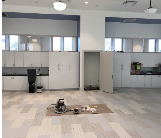
Lloyd Hall is looking good with new flooring, lights, cabinetry, and more
